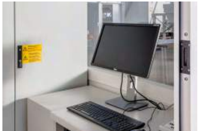
Integrated container with plant control system.
