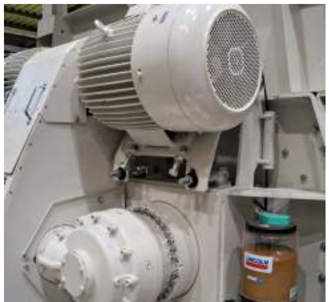
Mixer drive with automatic central greasing system.
